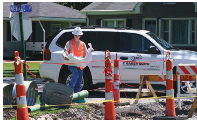
Construction Management - Project representation of drainage improvements in the city of Thibodaux
