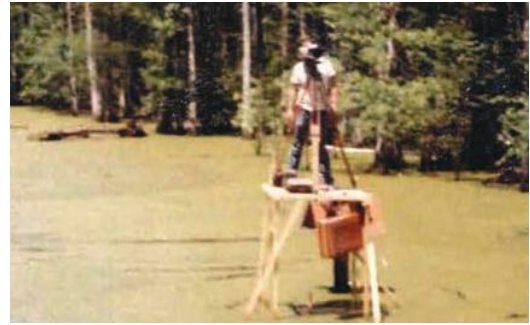
TBS instrument man set up on a hand made survey tower along a pipeline through a swamp
