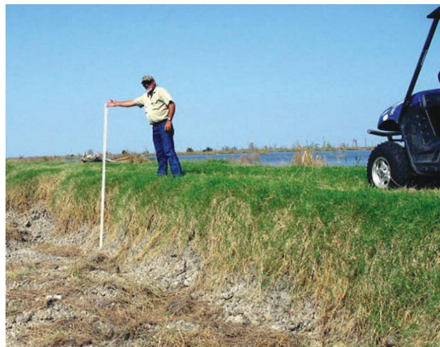
Danny Richard, TBS Party Chief, performing a levee damage survey
