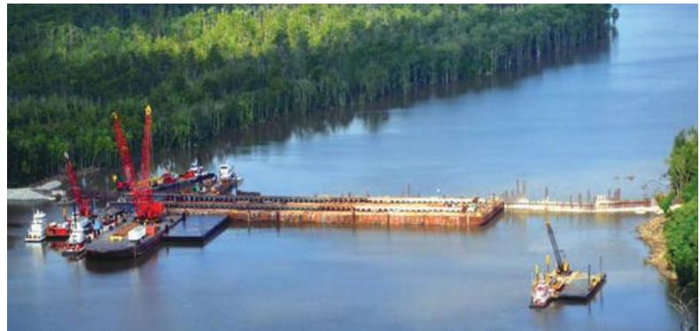
Barge and wing wall structure being installed in Bayou Chene to prevent backwater flooding
